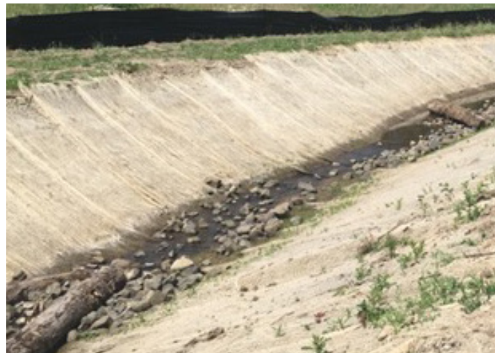
Bank protection was installed when the channel was dry before planting shrubs.
