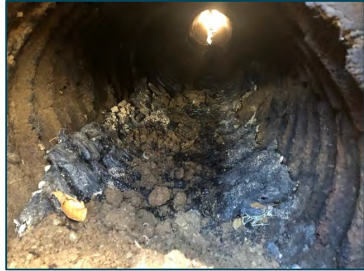
Photo 5. Burned out culvert
