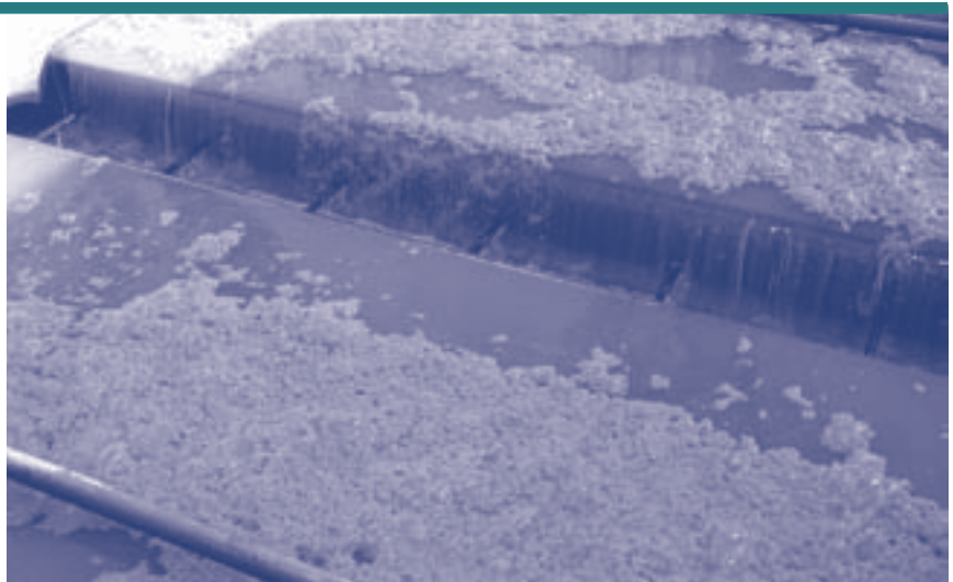
Rapid rate filter at Longview being backwashed following an inspection.
