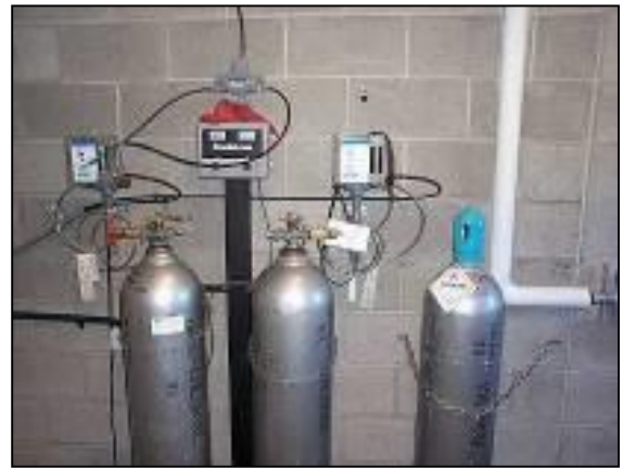
Gaseous chlorine cylinders
