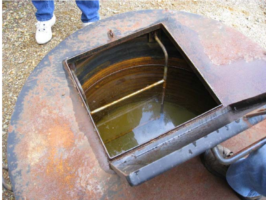
Figure 6. Open, water-filled manhole at main Formosa adit (June 10, 2008)
