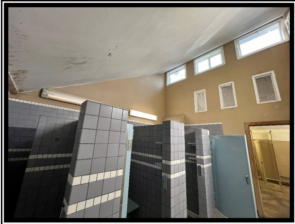
Figure 4 – Aging fixtures and finishes, difficult to maintain and clean.
