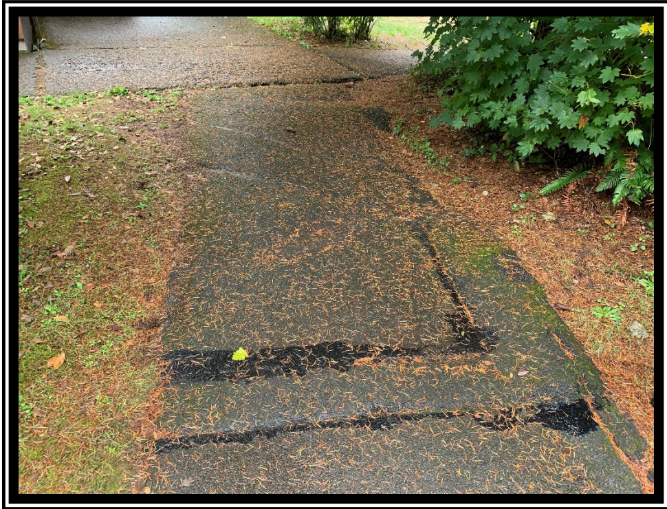
Figure 5 – Patches in paving, non-ADA path
