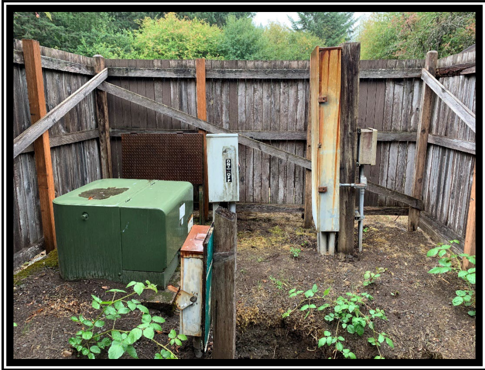
Figure 3 – Electrical and plumbing equipment in need of replacement.
