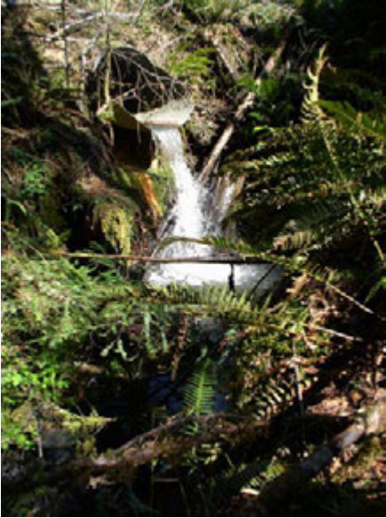
Top: This pre-project photo of the Seneca Jones TC culvert on Ben Branch Creek shows the seven-foot outfall that blocked all fish passage.
