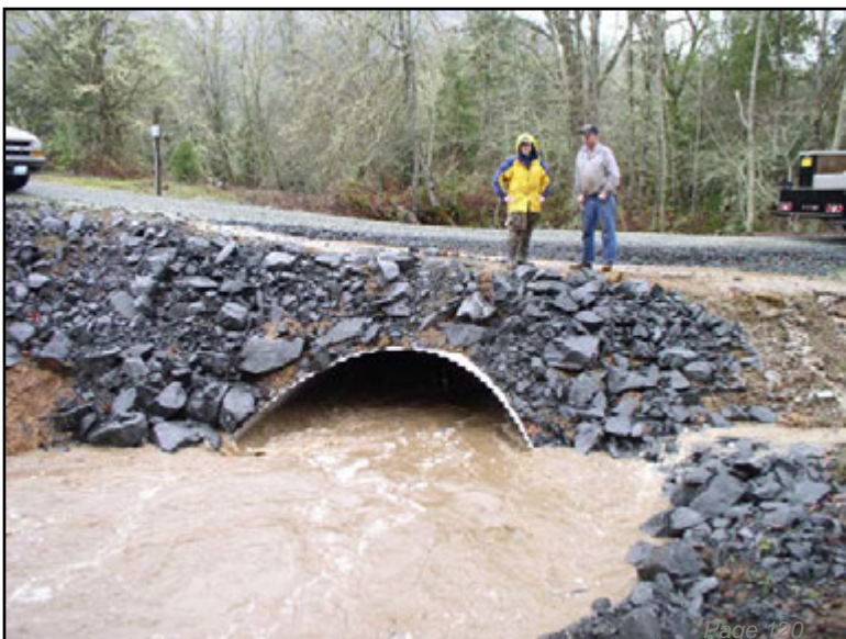
Bottom: This culvert, located on Gary Brownson's property, is shown during the December 2005 flood. Seneca Jones TC road crew installed this pipe and the one pictured above. With a BLM pipe replacement between these two, fish now have access to the entire length of Ben Branch Creek, a tributary to S. Myrtle Cr.
