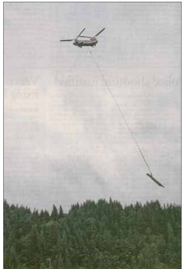
BELJAMIN SPINA/THE OREGONIAN A Columbia Helicopters Inc. helicopter puts a log into place this week as part of a project to reconnect and restore side channels of the Salmon River off U.S. 26 west of Zigzag. The logs re-create logjams that provide crucial refuge for imperiled salmon and steelhead.
