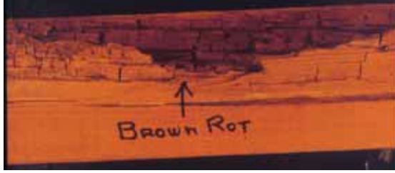
Figure 4. The final stage of wood decay by the brown rot can be identified by the dark brown color of the wood, excessive wood shrinkage, cross-grain cracking, and the ease with which the dry wood substance can be crushed to powder.
