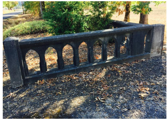
Sections look similar to the bridge rail from the Cape Creek Bridge
