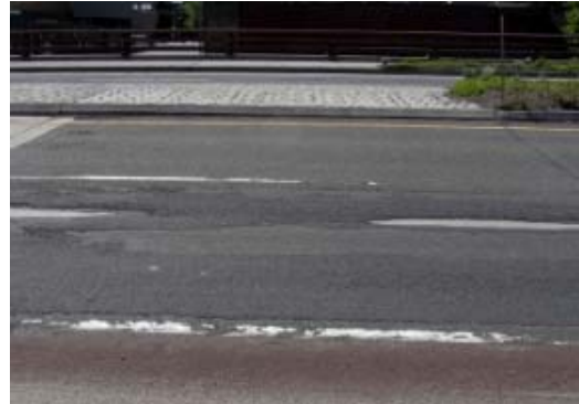
Rutting on the Bend Parkway (US 97).
