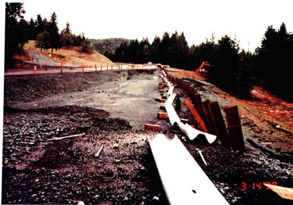
LANDSLIDE DISTRESS: MARCH 14, 1990
