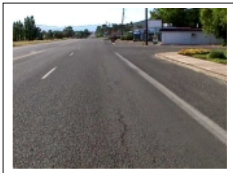
#34 Cracks in front of VRB Bank
