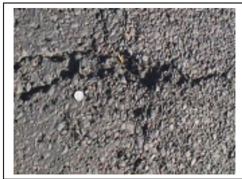
#33 Close-up of cracks near Compass Rose Store
