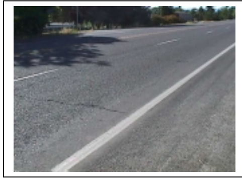
#32 4 transverse cracks near Compass Rose Store
