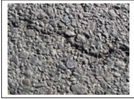
#36 Close-up of crack in front of VRB Bank
