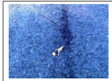
#18 Raveled area with crack.
