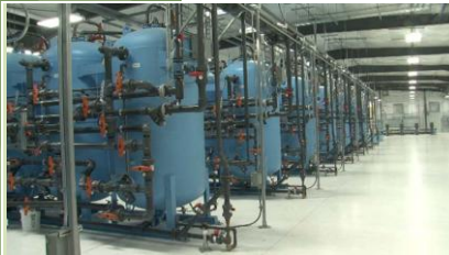
Inside a pump-and-treat facility at Hanford's 100-H Area, near the Columbia River.
