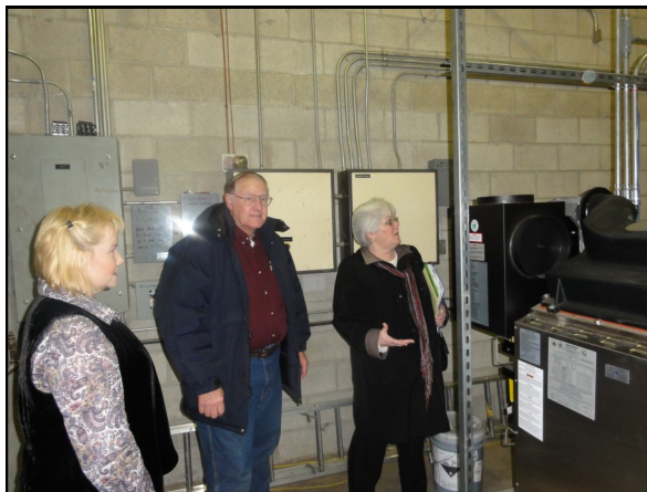
Rogue River Maintenance Supervisor James Charleboix, center, shows Lisa Marston, left, Rogue Valley Council of Governments, and Shanda Shribbs, Oregon Department of Energy Project Manager, the new Rogue River High School natural gas boilers installed with federal stimulus money.
