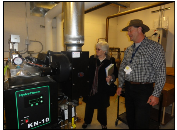
Grants Pass Maintenance Supervisor James Lowe, right, shows Shanda Shribbs, Oregon Department of Energy Project Manager, the new Parkside Elementary School natural gas boilers installed with federal stimulus money.
